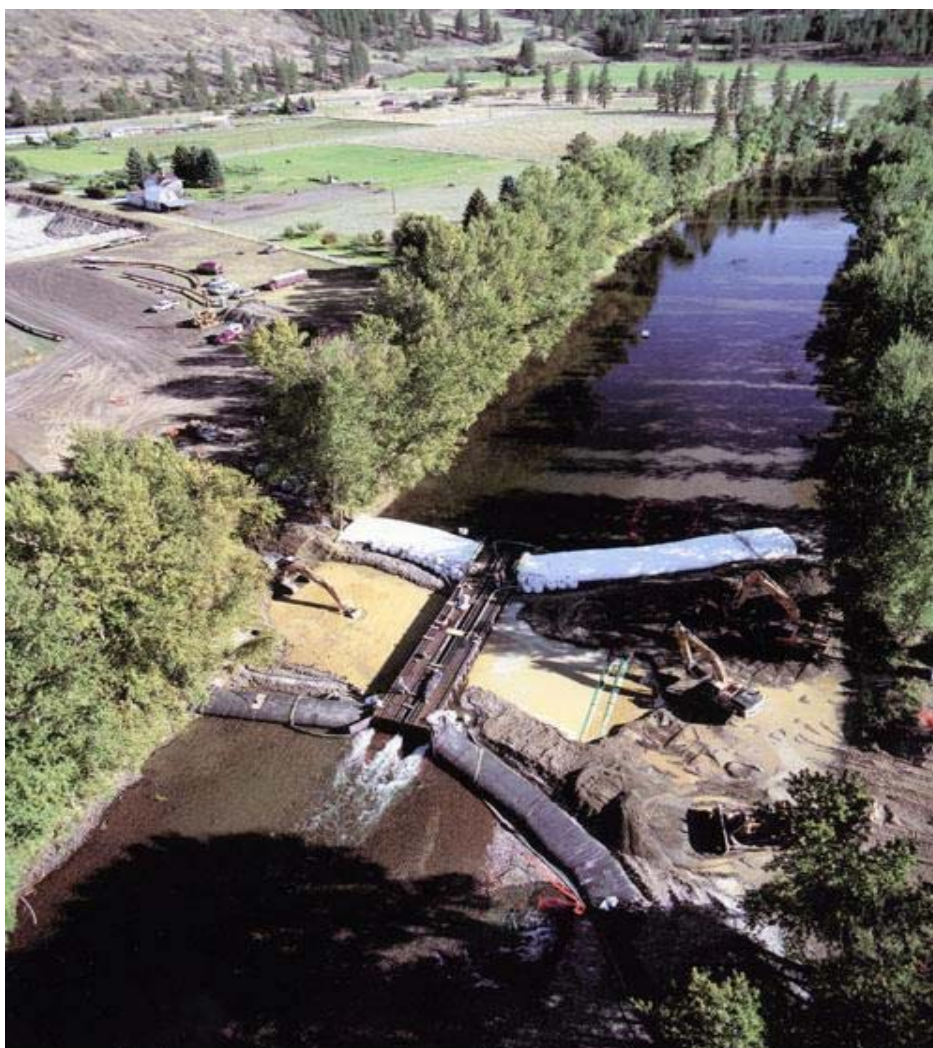
8' high X 200' long upstream, 4' high X 200' long downstream Double Superflume Crossing Kettle River, Grand Forks, BC
